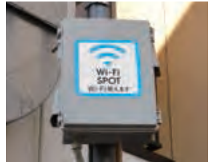
Wi-Fi ACCESS POINT
