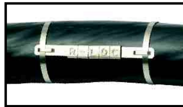
Marker Tags Installed on Power Cable
