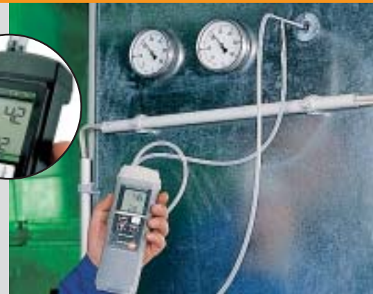
Measures flow with a Pitot tube in a ventilation duct
