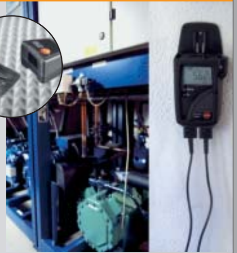
Measurement of air inlet and outlet temperature in refrigeration units
