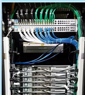
Computer room wiring
