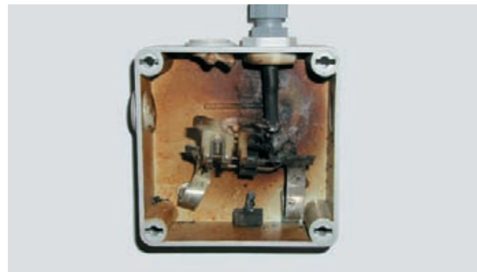
Module box after lightning strike
