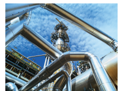
Chemical, Oil and Gas
