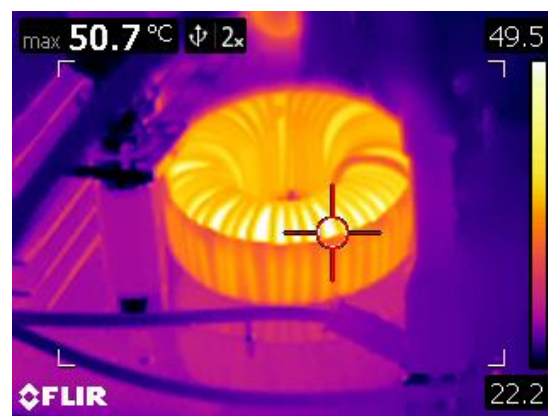
Figure 22. Thermal Scan of Inductor
